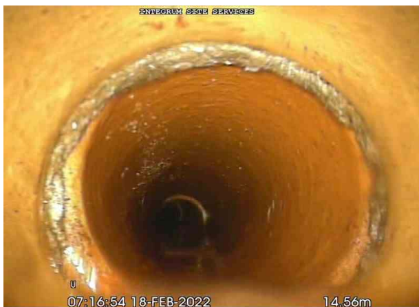
1-1-6A, 00:10:25, 14.50 m Joint displaced, medium
