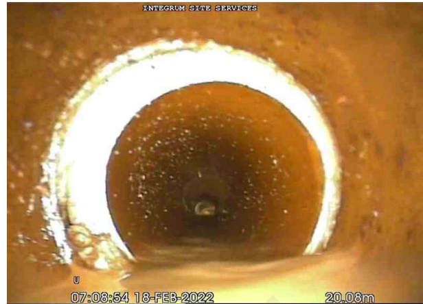
1-1-11A, 00:02:31, 20.08 m Joint displaced, large
