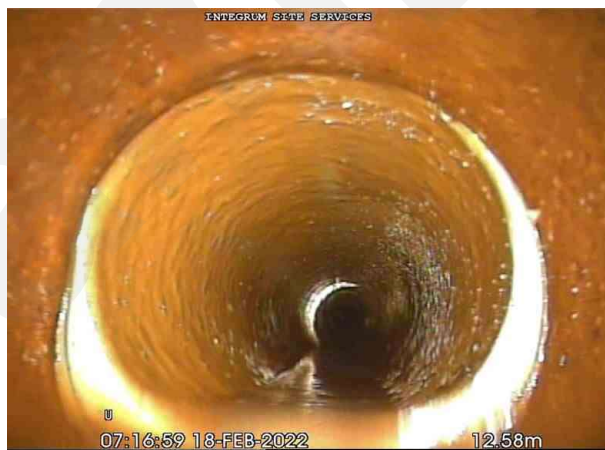
1-1-5A, 00:10:31, 12.80 m Joint displaced, medium
