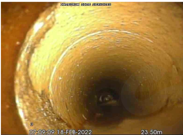
1-1-12A, 00:02:46, 21.00 m Pipe material changes to another material at this point, Appears to change to patch liner
