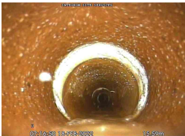
1-1-8A, 00:10:22, 15.59 m Joint displaced, large
