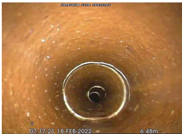
1-1-4A, 00:10:53, 6.47 m Fracture, circumferential from 9 o'clock to 5 o'clock
