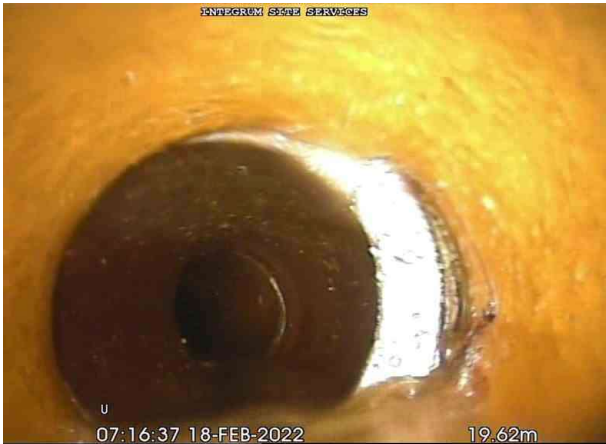
1-1-10A, 00:10:08, 19.62 m Joint displaced, large
