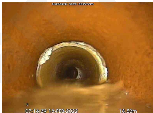
1-1-9A, 00:10:10, 18.53 m Joint displaced, large
