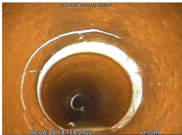
1-1-3A, 00:00:25, 0.75 m Fracture, circumferential from 7 o'clock to 1 o'clock
