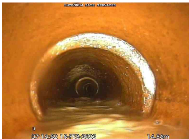
1-1-7A, 00:10:24, 15.20 m Joint displaced, medium
